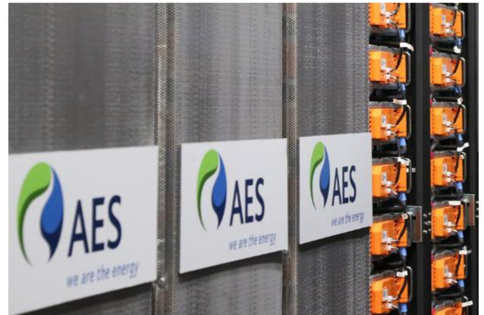
Batteries as part of an AES 'Advancion'-branded utility-scale installation. Image credit: AES
